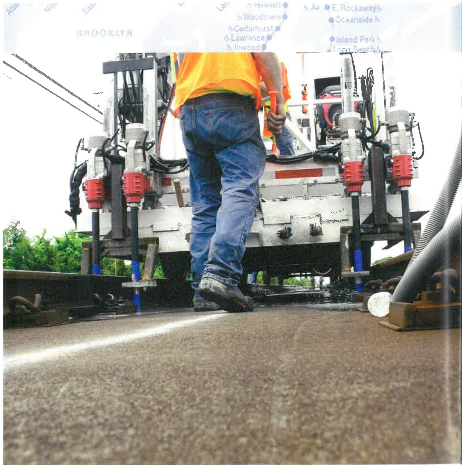
The LIRR Railcar allowed the drilling team to create four core holes at one time.
